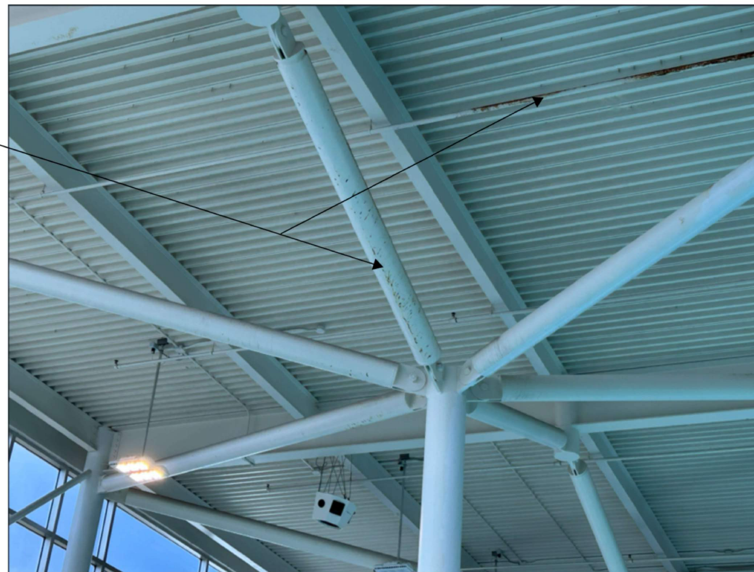
FIGURE 2: RUST STAIN ON BRACINGS AND ELECTRICAL CONDUIT SCALE: N.T.S
