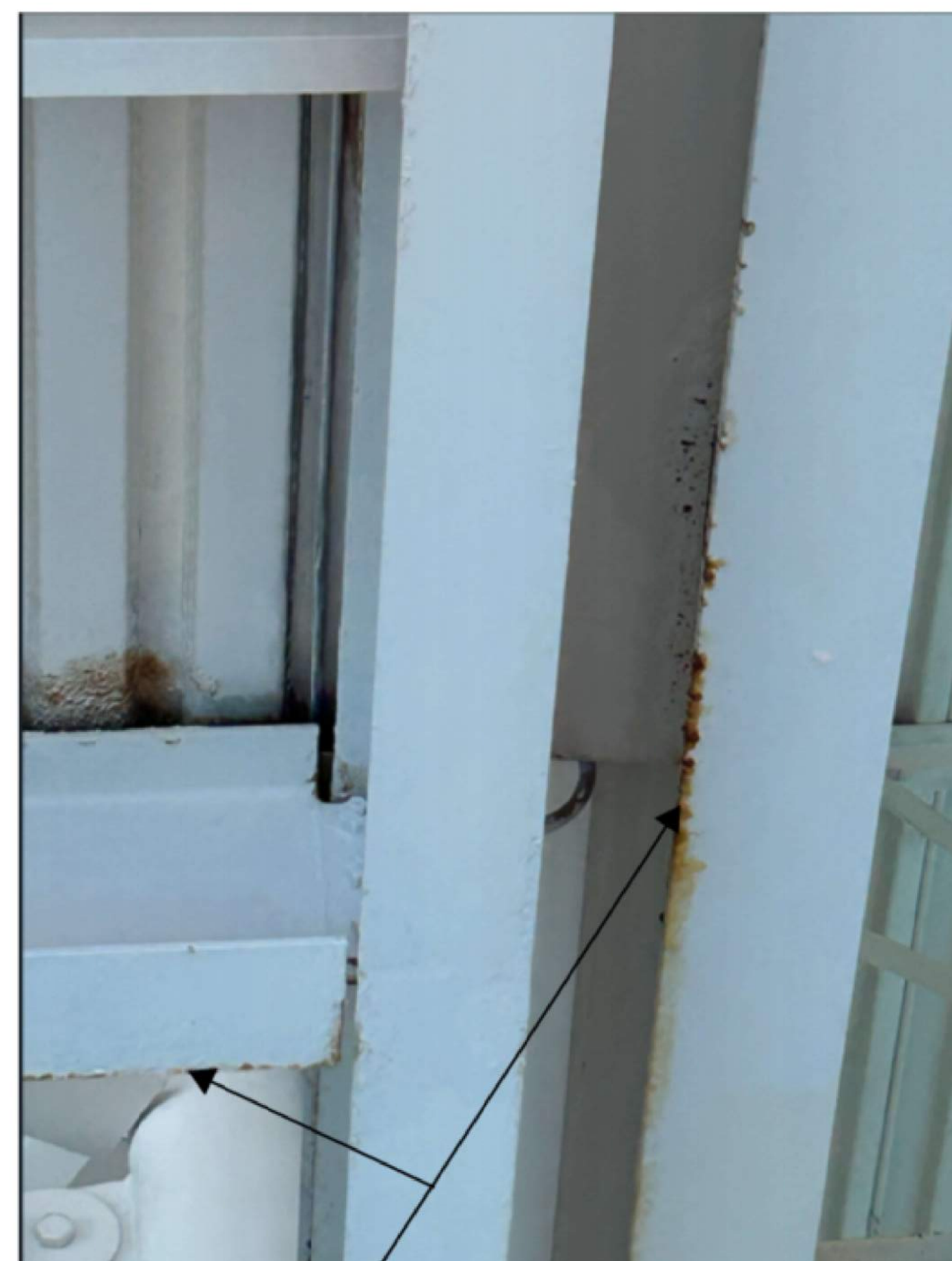
WIRE BRUSH AND EPOXY PAINT TO MATCH EXISTING, ALL RUST ON EXISTING WATER SLIDE PLATFORM FRAMINGS.
