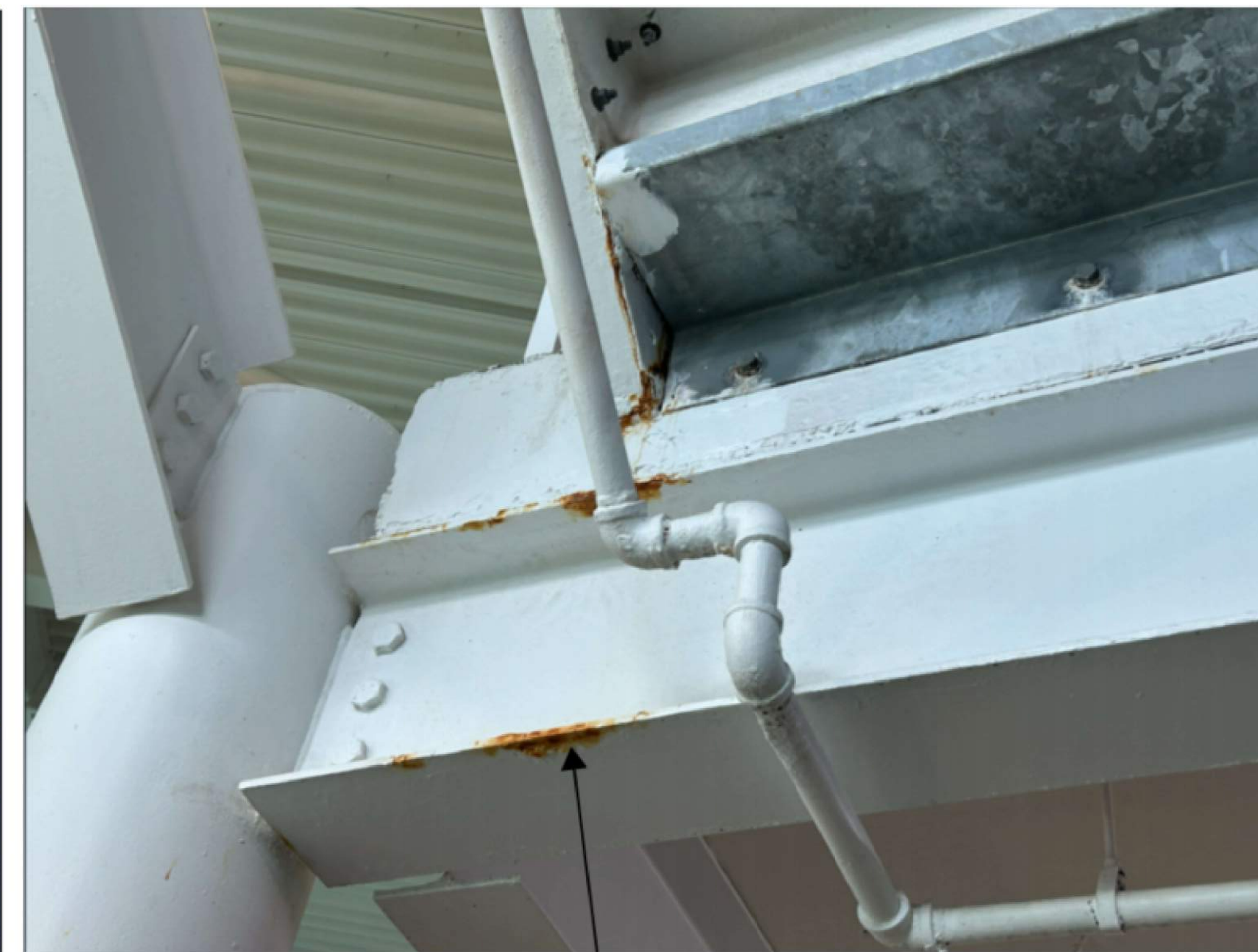
WIRE BRUSH AND EPOXY PAINT TO MATCH EXISTING, ALL RUST ON EXISTING STEEL FRAMINGS.
