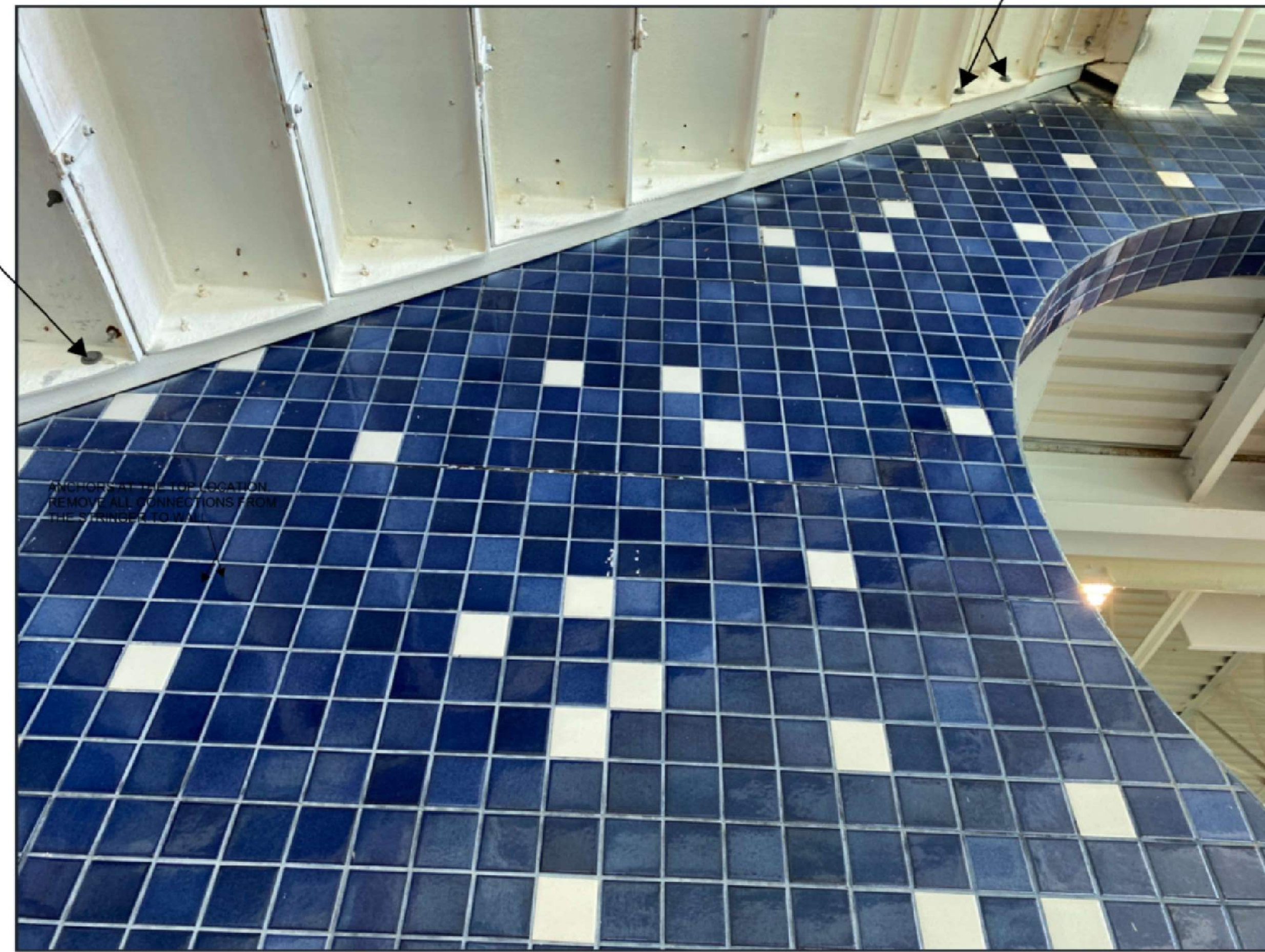
FIGURE 8: VIEW SHOWING THE CMU FEATURE WALL, SOFFIT OF THE WATERSLIDE PLATFORM STAIR AND ANCHORS SUSPECTED TO BE FASTENED TO THE WALL
