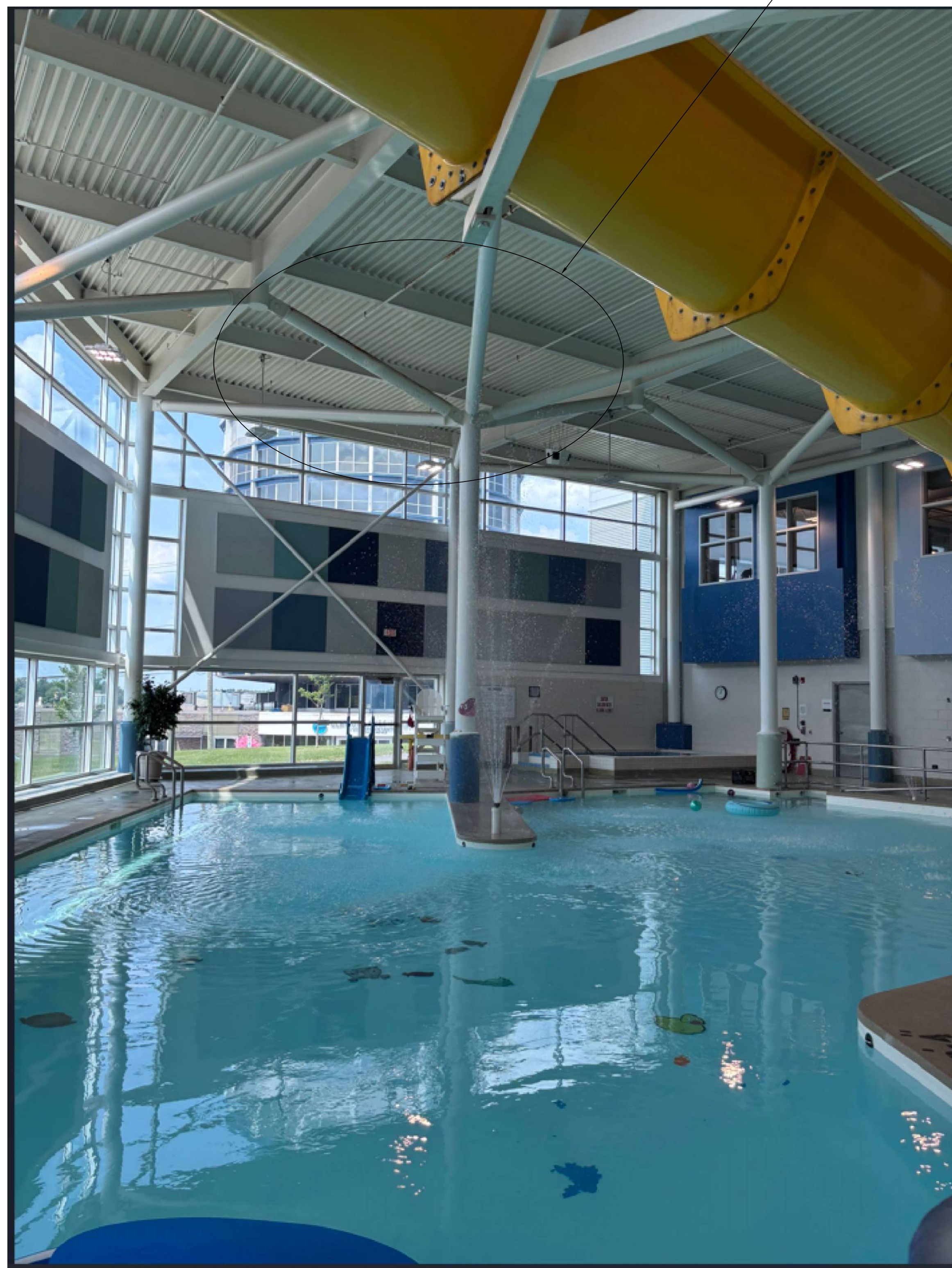
FIGURE 1: VIEW SHOWING AN AREA SAMPLE OF RUST LOCATION ON COLUMNS, BRACINGS AND ELECTRICAL CONDUIT.
