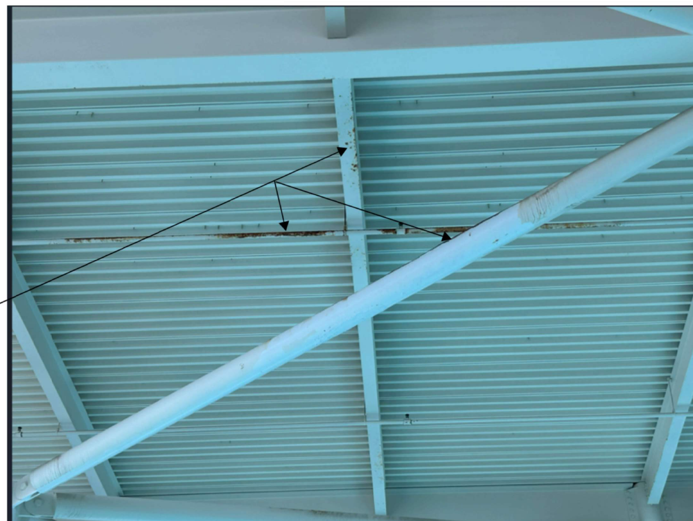
FIGURE 3: RUST STAIN ON STRUCTURAL STEEL, BRACING AND ELECTRICAL CONDUIT SCALE: N.T.S
