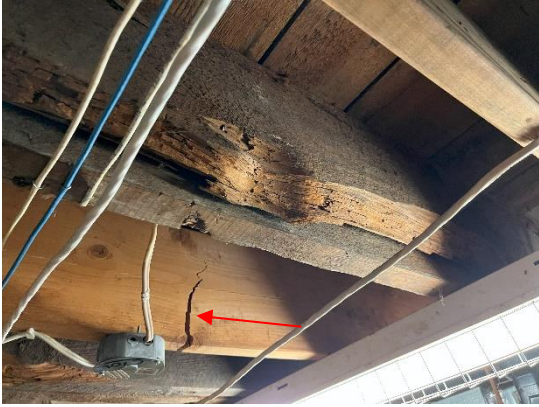
Figure 25: Joist deteriorating observed at various joists.
