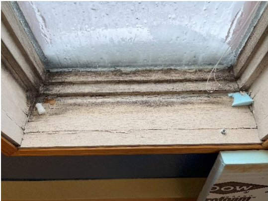
Figure 13: Mold growth and deterioration of interior windowsill and jamb finishes.
