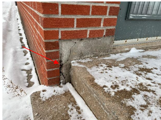
Figure 38: Delaminating observed at southeast corner of concrete foundation wall.
