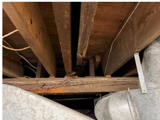
Figure 24: Beam supported by concrete columns observed to be stressed.
