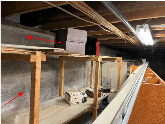
Figure 35: Some minor cracking observed at the south elevation foundation wall.
