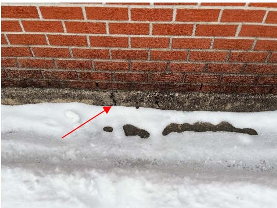
Figure 37: Some minor cracking observed at the exterior of the south elevation foundation wall.
