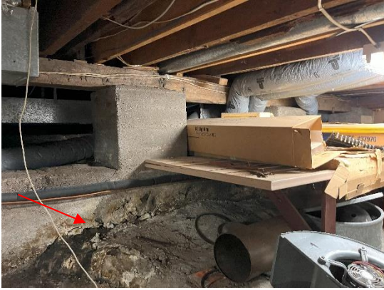
Figure 33: Some delamination of the concrete skim coat and cracking in the concrete footings.
