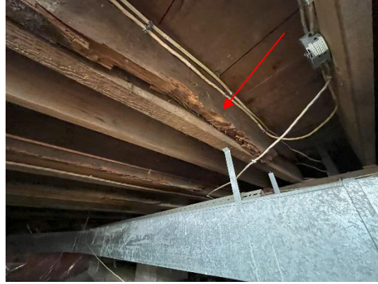
Figure 26: Bottom of joists were observed to be damaged at multiple locations. Some joists appear to have been sistered together.
