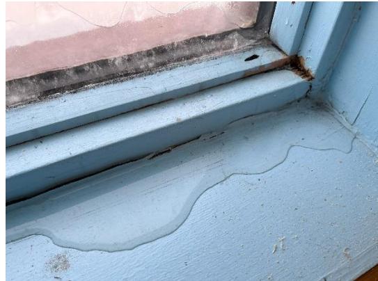
Figure 14: Large amounts of water pooling at the interior windowsills.
