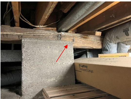
Figure 23: Wooden beam observed to be notched into concrete column.
