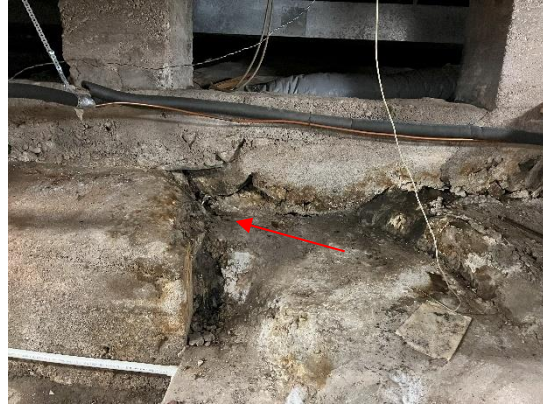
Figure 34: Some delamination and cracking in the concrete footings.
