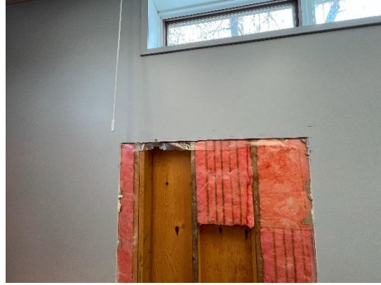
Figure 06: The Stud cavities were generally observed to be filled with R-20 Batt insulation.
