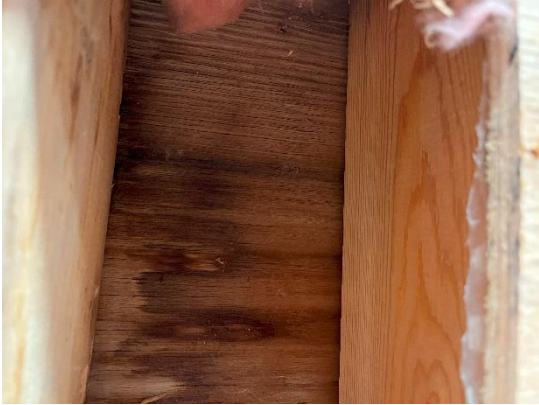
Figure 11: The plywood sheathing was observed to be stained at interior opening #3.
