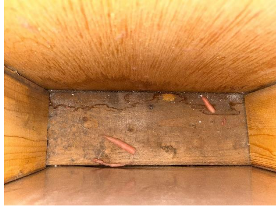
Figure 12: Evidence of previous moisture staining observed at bottom plate and base of sheathing.
