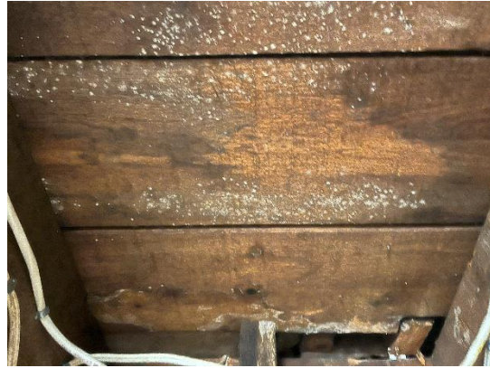
Figure 28: Dry rot observed in isolated location.
