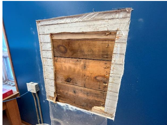
Figure 10: Opening 4, completed at the north wall exposed tongue and groove ship lap over wood plank. Condition of wood studs were not confirmed.
