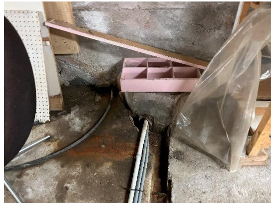
Figure 36: Evidence of moisture at the floor appears to be concentrated near assumed sump pump.
