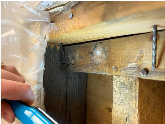
Figure 09: Organic growth in wall framing at older condition framing.
