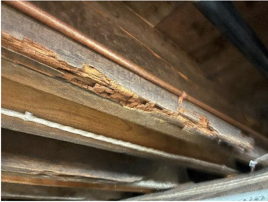
Figure 27: Joist appears to be deteriorating and stressed.
