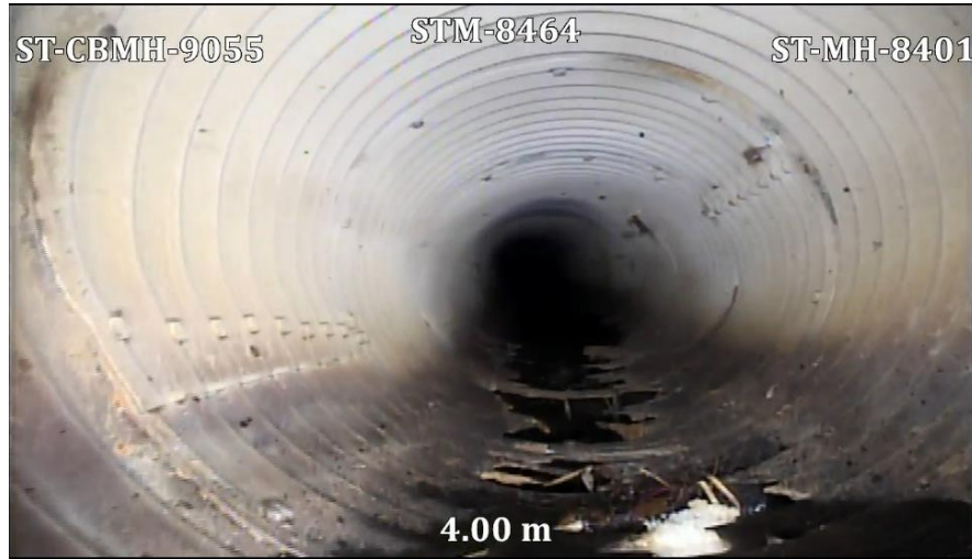
Figure 1: Deteriorated Storm Piping
