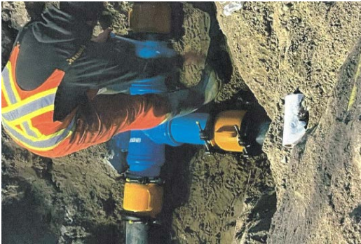
Outen Lane water main break
