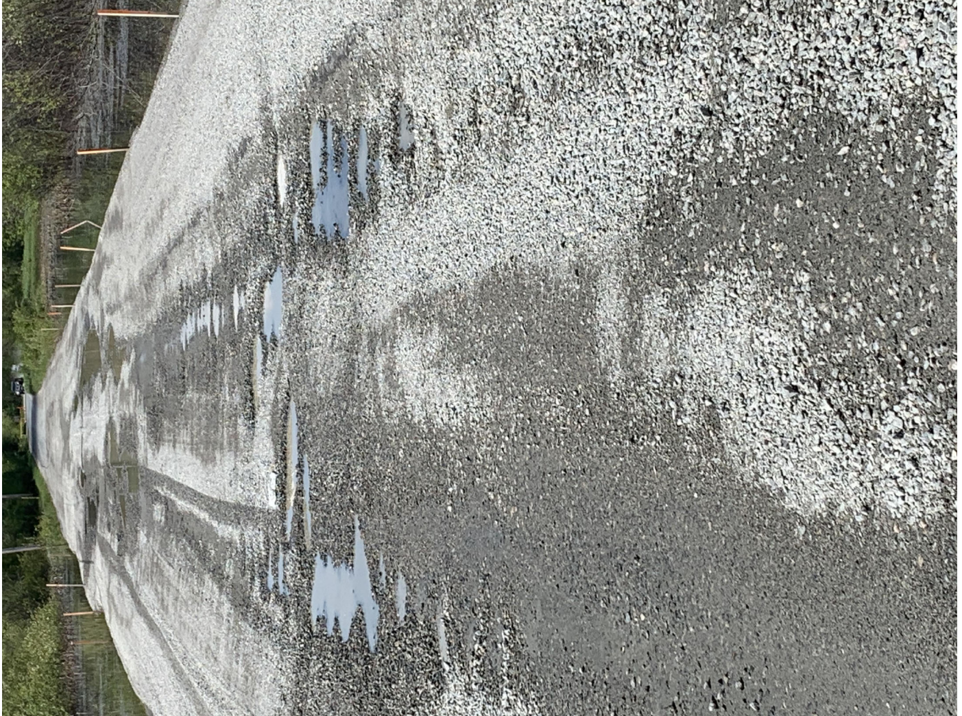
C:\Users\rwilcott\Pictures\2022 Flooding photos\Hooterville Trail Centre section June 9-2022.jpg
