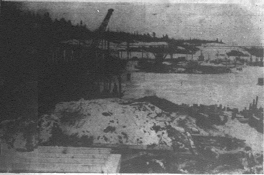
Steady progress is being made on the construction of the new Hospital Bridge. Here is a recent M & N photo showing one view of the project.
